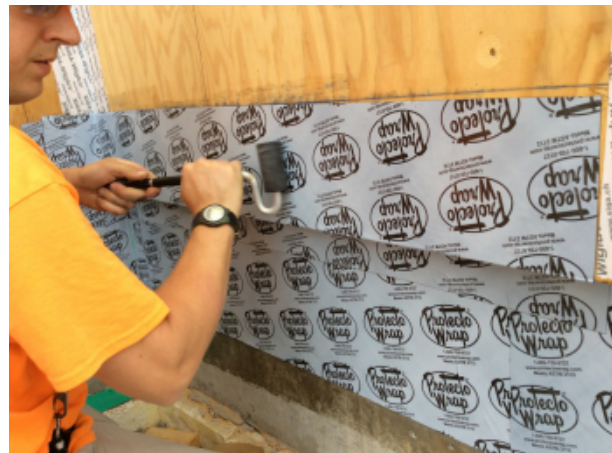
Fig. 21 - A laminate roller is used to apply pressure to the SAM to help ensure adhesion to the substrate and eliminate air pockets and pinhole leaks.
