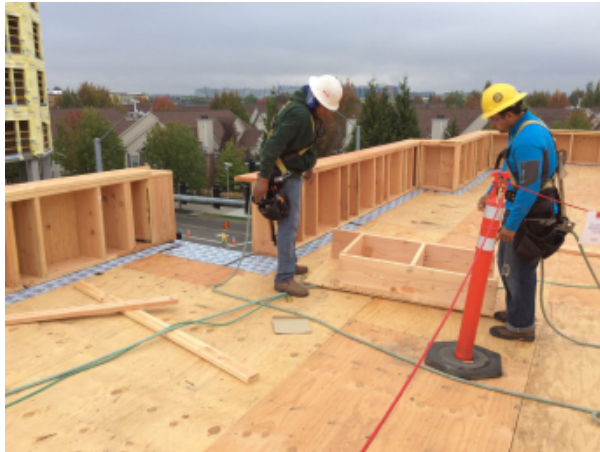
Fig. 58 - Parapet wall framing is installed over the SAM transition seal. SAM extends several inches outward from the inside of the parapet to facilitate the tie-in with the SAM vapor barrier / air barrier that will be installed later over the roof sheathing.
