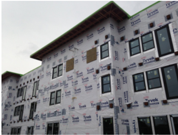
Fig. 48 - View of exterior walls after completion of the water-resistive barrier system. Treated wood blocks have been installed over the WRB at balcony ledger locations. Saddle flashing is to be installed over each block.
