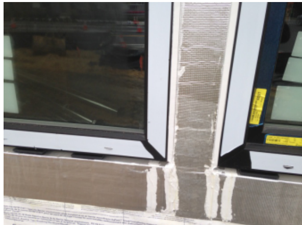
Fig. 45 - Water seal at exterior perimeter of windows. These seals occur at the jambs and head of each window. The sill is left open to allow free drainage from the sill pan area.
