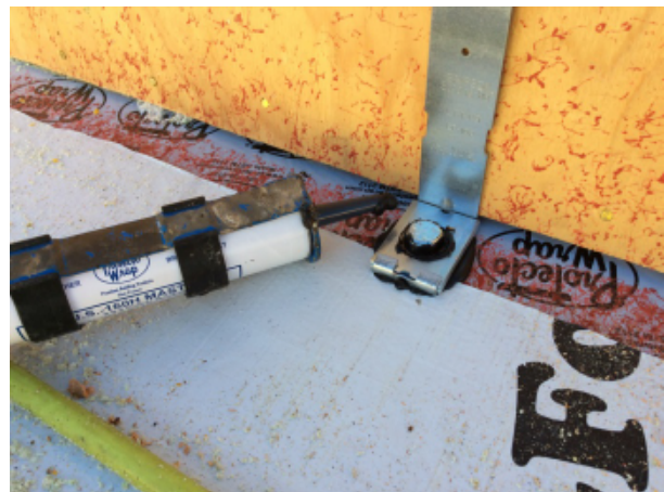
Fig. 61 - Steel strapping with large lag screws required to tie the parapet framing to the roof truss framing. These large penetrations are sealed to ensure air barrier continuity.
