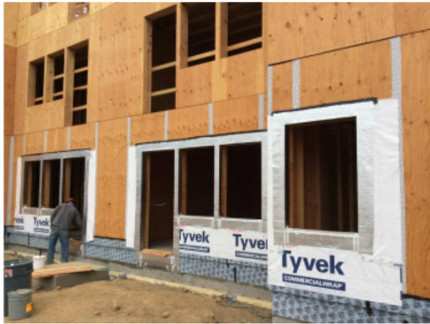
Fig. 32 - View of typical rough opening preparation at ground floor units, showing ganged windows and exterior door. This view also shows the SAM flashing and air seal applied at the base of wall.
