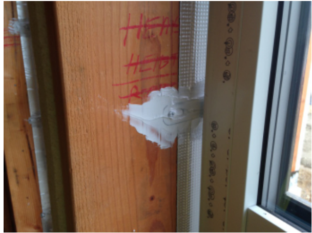
Fig. 43 - Sealant applied to strap anchor after fastening. Backer rod and sealant is subsequently installed in the gap between SAM flashing and window frame.
