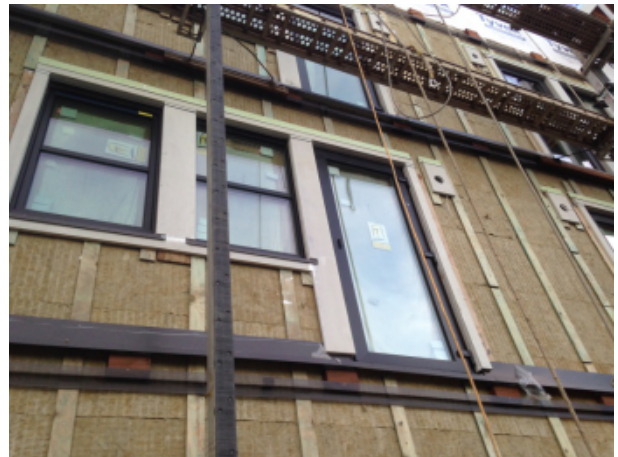
Fig. 51 - View showing trim installed prior to siding installation. Flashing and ventilation trim associated with the balcony ledger can be seen at the floor line area.
