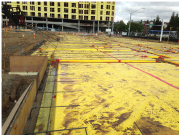
Fig. 18 - When a significant amount of rainfall occurred just prior to one of the slab pours, the team was relieved the vapor barrier had been moved to the top of the Insulation.
