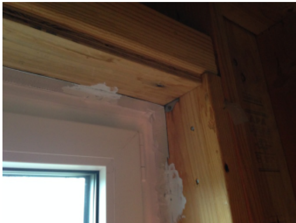
Fig. 44 - Air and water seal at interior perimeter of window. This seal completes the air barrier continuity from the wall to the window.
