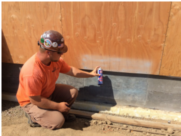
Fig. 20 - Primer is applied to the concrete prior to installation of the SAM.
