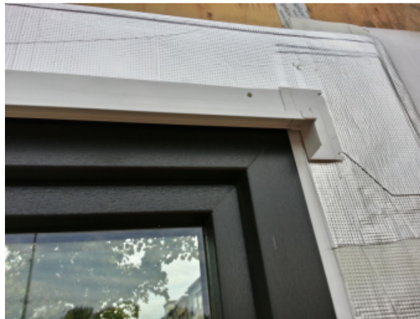
Fig. 47 - Head flashing is installed directly above the window frame. WRB from the wall area above the window is then folded down to lap over the head flashing.
