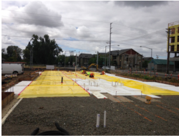
Fig. 16 - Sub-slab insulation is installed over the gravel base. Vapor barrier installation follows.
