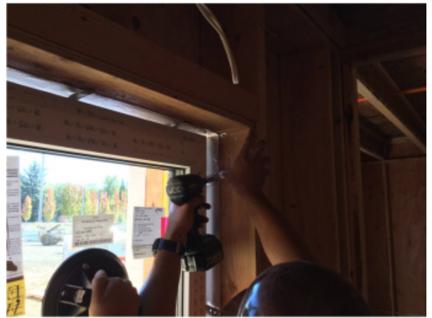
Fig. 37 - Window is fastened at the jambs and head using strap anchors provided by the window manufacturer.
