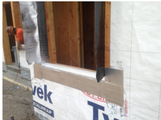
Fig. 27 - Sill pan flashing is complete. SAM flashing is applied to the jambs. SAM primer is applied to all substrate materials prior to adhering the SAM.
