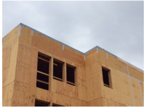
Fig. 57 - SAM seal is applied to the top of "the box." Note the poly sheeting to the right. It has been placed temporarily to keep the sheathing dry prior to installation of the membrane.
