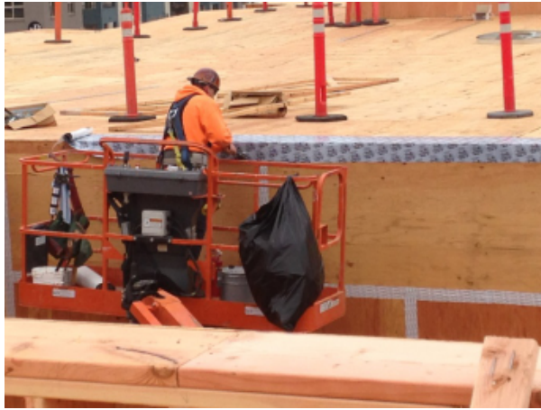
Fig. 56 - SAM is applied to interface between wall and roof. This essentially completes the seal of "the box" by connecting the wall sheathing to the roof sheathing.
