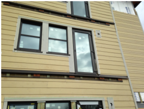
Fig. 52 - View showing similar balcony area with siding installed. Balcony ledgers will be attached to the intermittently placed wood blocks. This allows for thermal barrier continuity at the floor line area.
