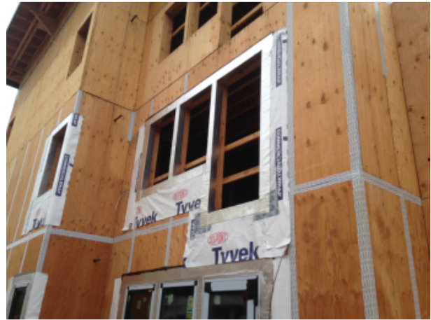
Fig. 33 - View of rough opening prep at upper floor units where balconies occur. The water-resistive barrier system will be installed and completed in its entirety prior to installing the balcony structure.
