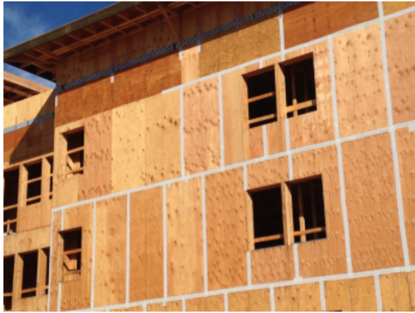
Fig. 24 - View of exterior walls prior to preparation of the window openings. The plywood wall sheathing serves as the primary air barrier material at the walls. All joints in the sheathing are sealed with tape.
