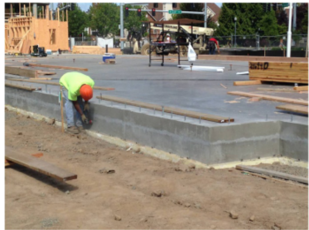
Fig. 19 - Grinding the concrete footing edge to provide a smooth and consistent substrate for application of the SAM flashing and air seal at the typical base of wall condition.
