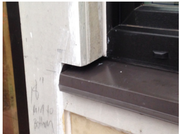
Fig. 53 - Metal sill flashing termination and fiber cement trim configuration at typical window.
