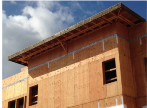
Fig. 59 - View of parapet walls framed on top of "the box." Once the joints in the wall sheathing are taped, the windows are installed and sealed, and SAM is installed over the roof sheathing, the air barrier system will be largely complete.
