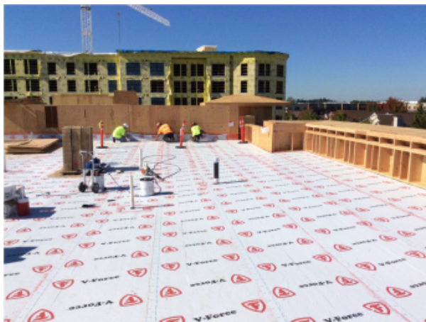
Fig. 60 - SAM vapor barrier / air barrier installed over the roof sheathing. The SAM also serves as a temporary roof prior to placement of the roof insulation, coverboard and TPO roof membrane.
