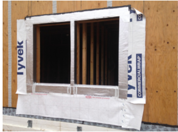
Fig. 25 - Typical rough opening preparation prior to window installation. Strips of WRB material are installed, then SAM flashing is used to wrap the openings for water management and airtightness at this crucial interface.
