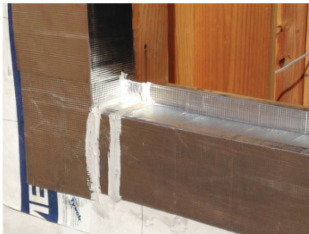
Fig. 28 - Detail view of sill pan flashing. The back leg of the pan is supported on the aluminum angle provided by the window manufacturer for attachment of the window sill.
