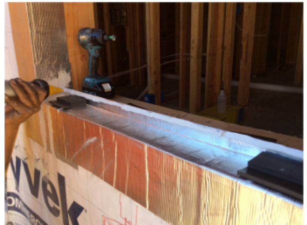
Fig. 35 - Sealant is applied to the back leg of the sill pan prior to setting window into opening.
