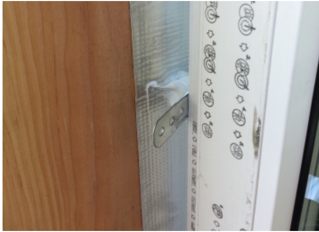
Fig. 42 - Sealant applied to strap anchor location prior to fastening. This is an important detail to encapsulate the anchor in sealant to prevent air leakage.
