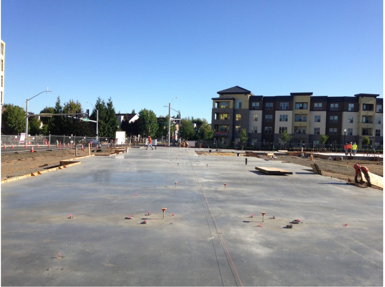
The finished slab at Zone 1 (west wing). Ready for snapping lines and raising walls!
