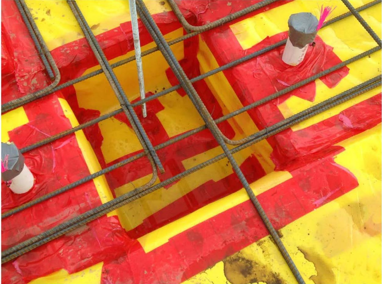
The foam was configured to provide for a few deep footings. These cavities filled with rainwater but we punched a few holes in the vapor barrier to drain the collected water and then sealed the holes prior to the slab pour.
