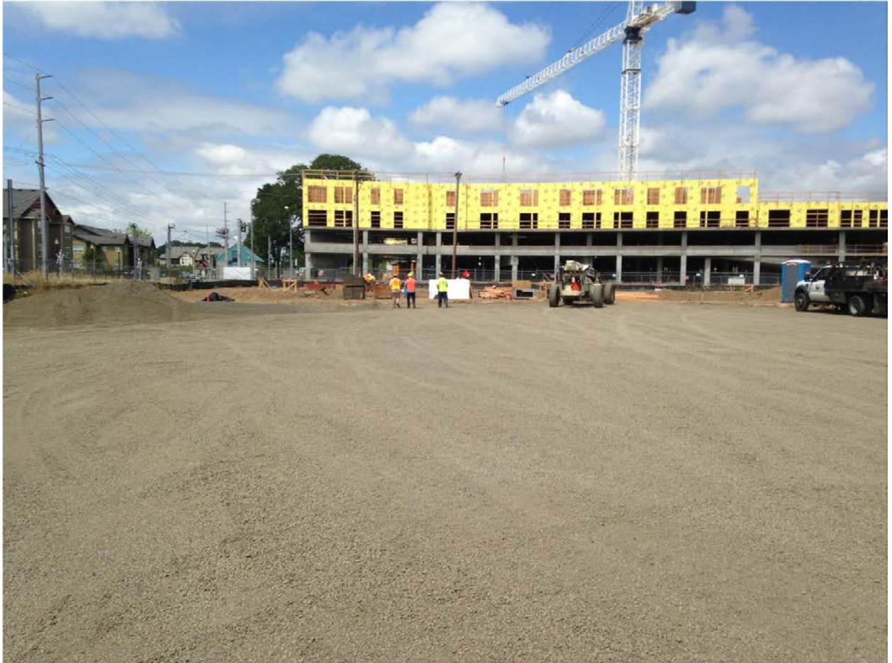
The site has been cleared and a rock pad placed to accommodate construction traffic. The building visible in the distance (to the west of our site) will be a mixed-use, market rate apartment building when completed in 2015.
