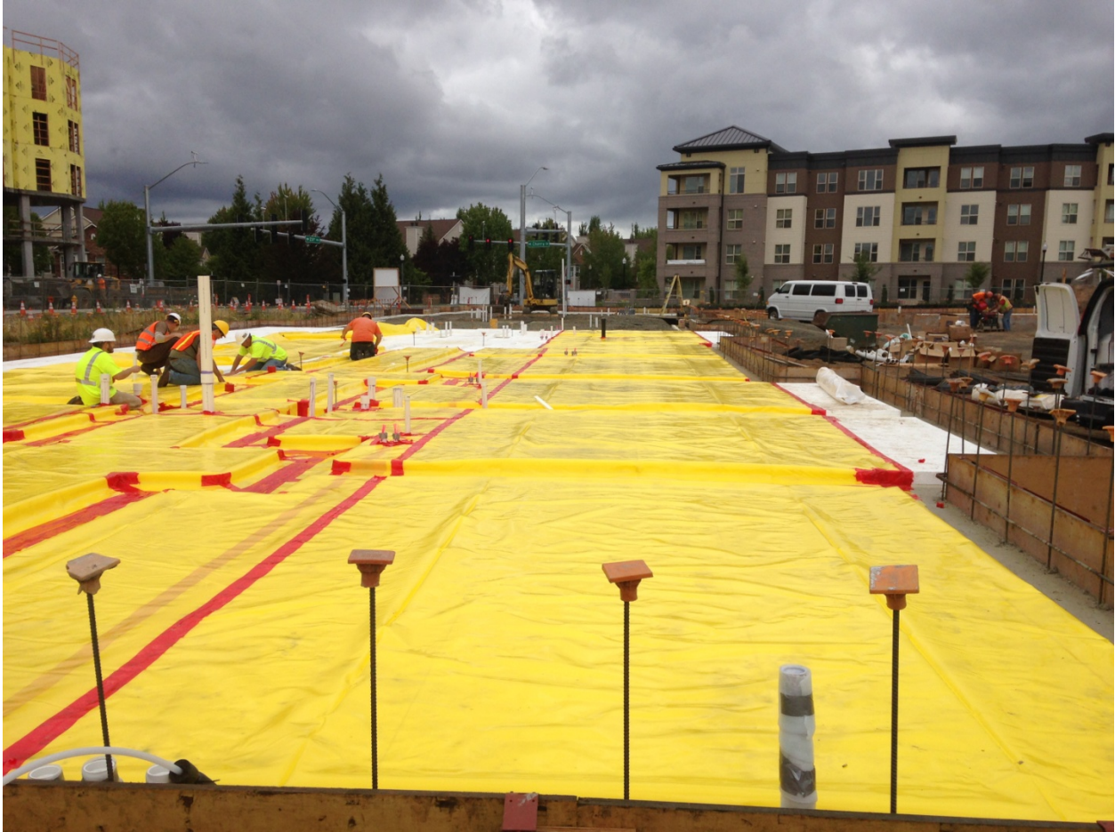
Vapor barrier installation begins at Zone 1. The vapor barrier is installed on top of the foam insulation, thus avoiding any potential to create a "pond" of water should it rain prior to the slab pour.
