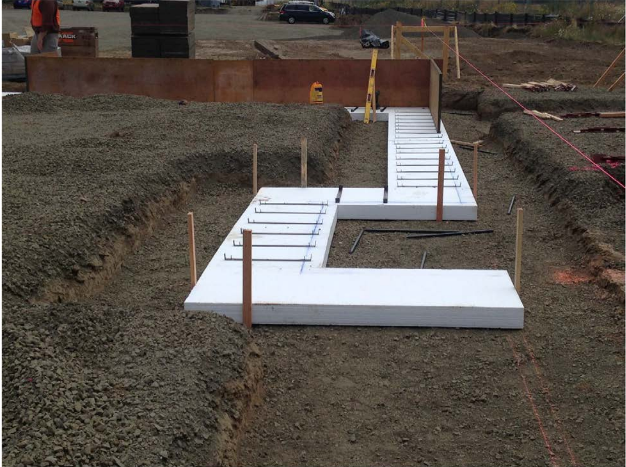
The building edge is laid out on the compacted and level gravel base installed over the subgrade, foam is placed, and work begins on the formwork for the perimeter footings.
