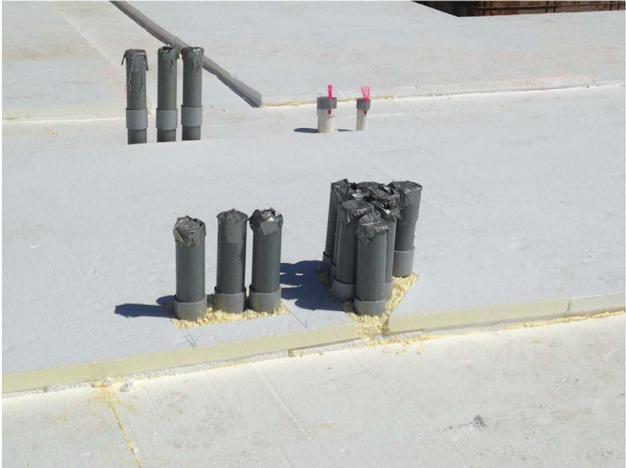
Spray foam is used at voids around penetrations of the slab insulation and at any locations where gaps occur in the insulation.
