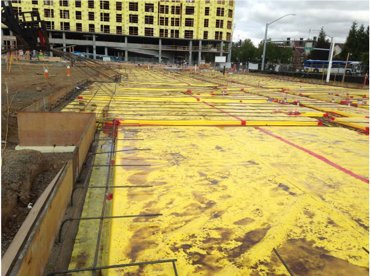
It never rains in Portland in August...but it did this year! Fortunately the water ran off to the sides of the assembly and the barrier surface was dry by the day of the slab pour.
