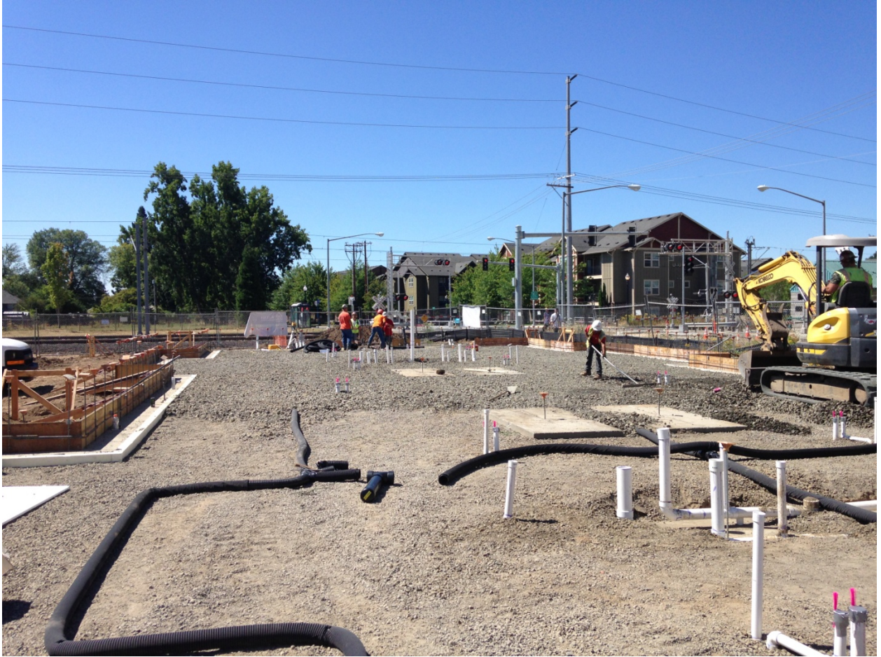
View of the west wing showing the underground plumbing pipes (white) and the beginning of the radon mitigation system installation (black pipes).
