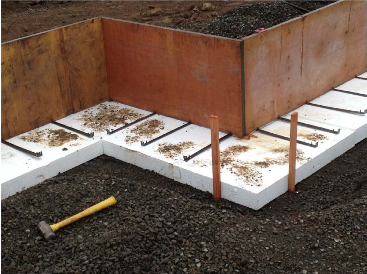
The foam sits firmly on the gravel base. Due to the excellent work by the excavation subcontractor, controlled density fill was not required.
