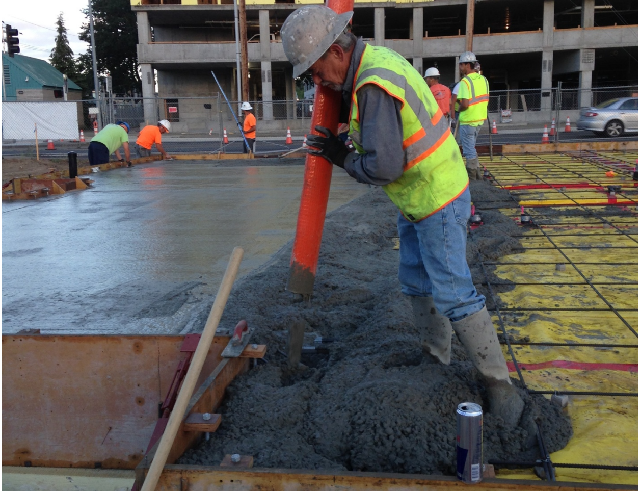
The "mud" (concrete) is pumped, placed over the vapor barrier, and finish work begins.
