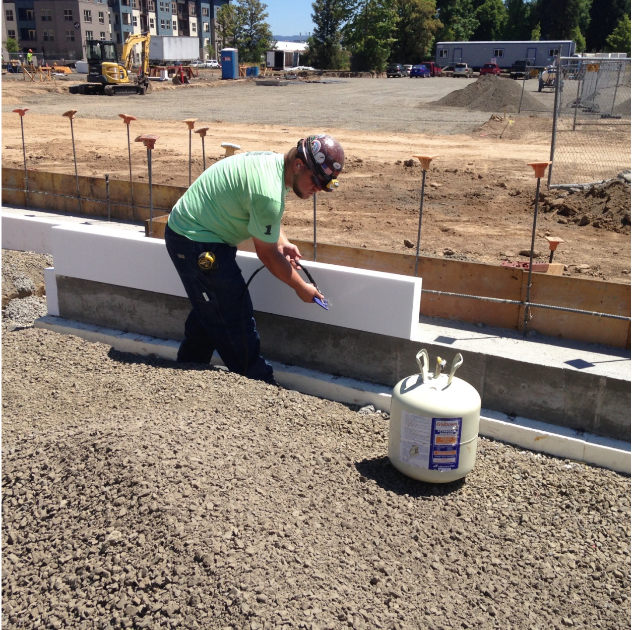
Nick applies adhesive to the foam which is then adhered to the footing.
