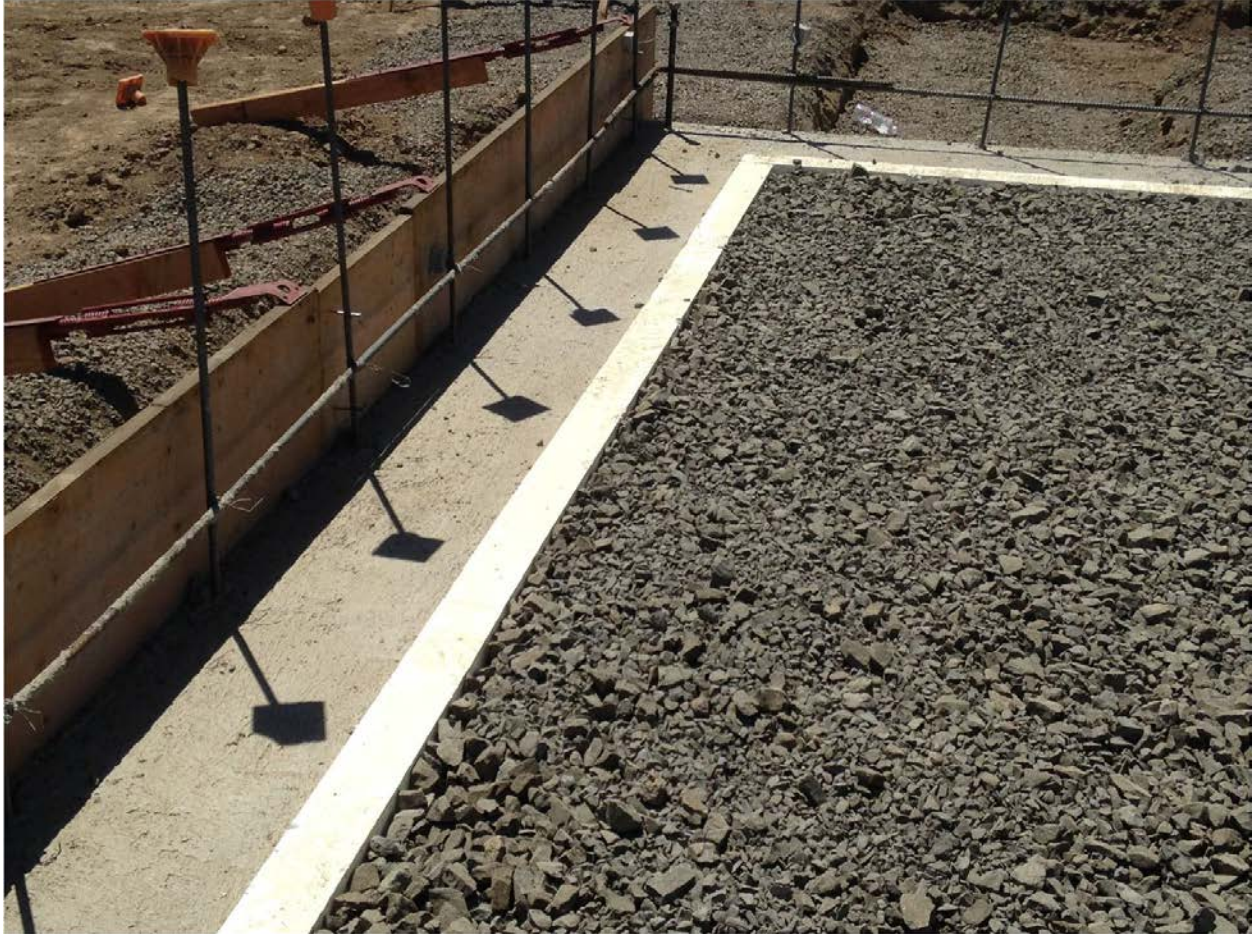
View of the crushed gravel base layer (containing radon piping), prior to installation of the slab insulation.
