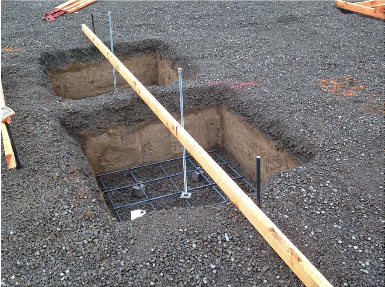
Excavation for "deadman" footings. A number of these footings provide restraint at points of high lateral load in the building.
