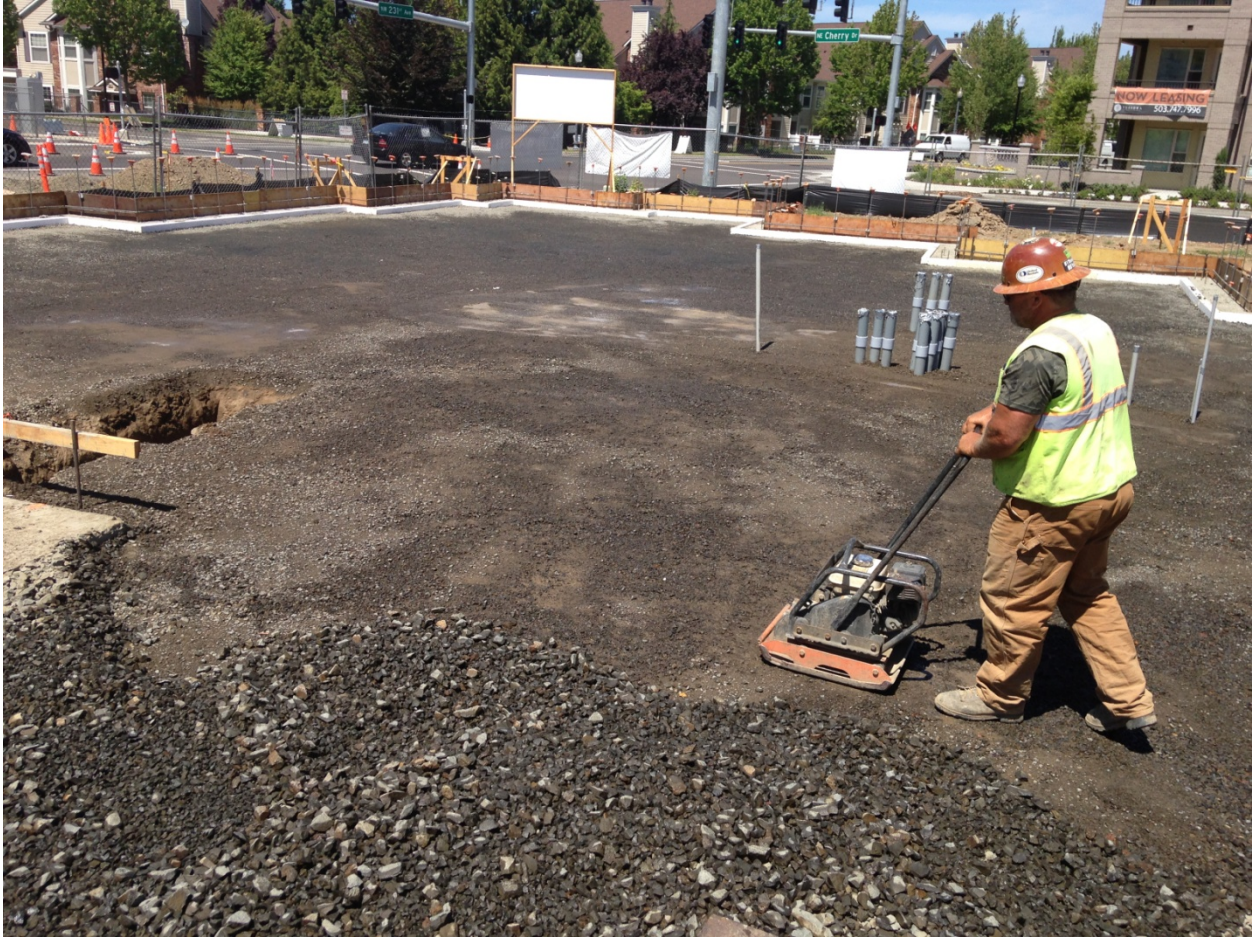
Compacting the gravel base for the foundation slab. On top of this base goes the radon mitigation system, the slab foam insulation layer, the vapor barrier, and then the concrete slab-on-grade.
