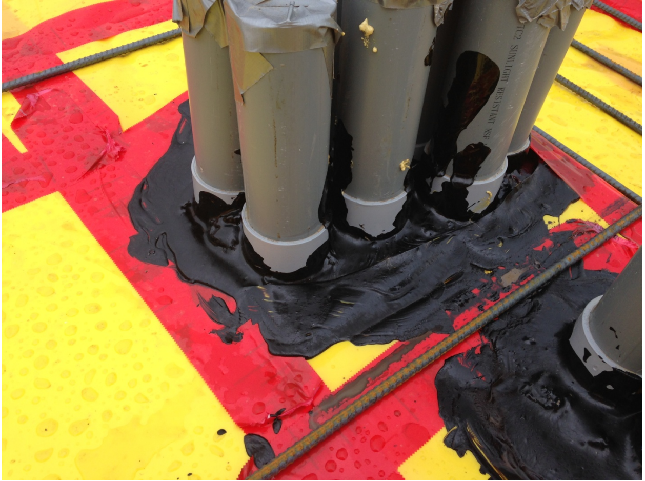
Where ganged conduits occur, the vapor barrier is sealed with a mastic accessory product.
