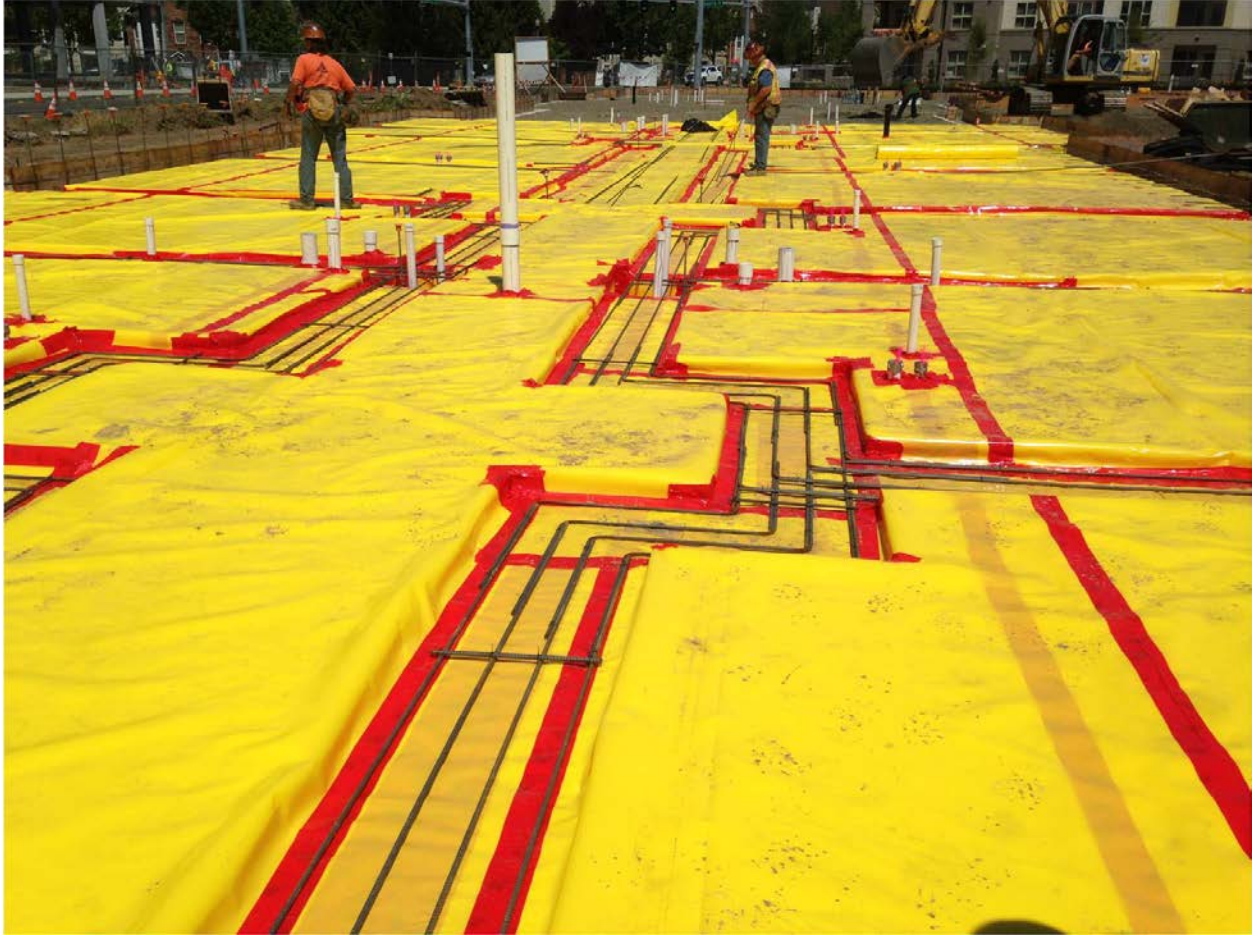
The vapor barrier is taped with manufacturer's sealing tape at all lap seams and penetrations.
