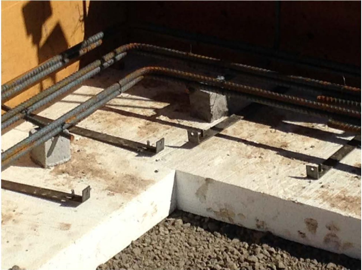
Detail view of foam insulation placed on gravel base prior to completion of the footing formwork. Note the tight joints and the firm placement on the compacted gravel base.
