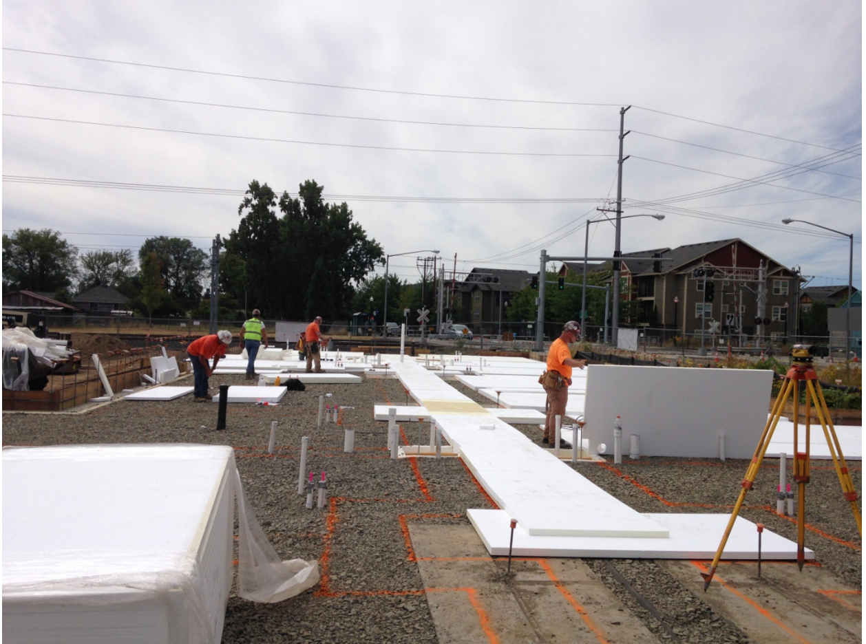
The first layers of EPS foam slab insulation are placed over the gravel base and the deadman footings. Note the layout markings on the gravel, denoting the thickened slab / interior bearing wall footing locations. 1" thick EPS will be placed in those locations.
