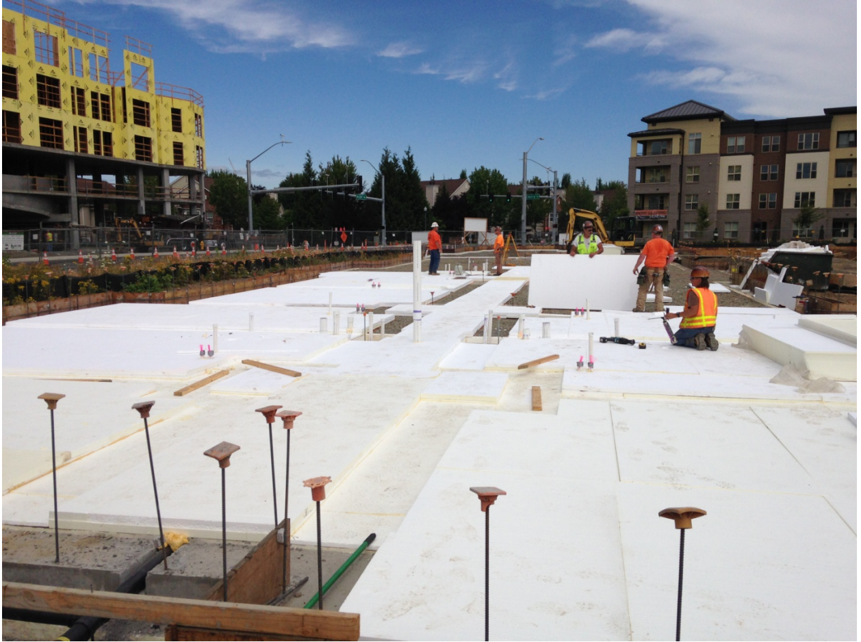
Foam insulation is cut and trimmed to fit around pipes and other slab penetrations.
