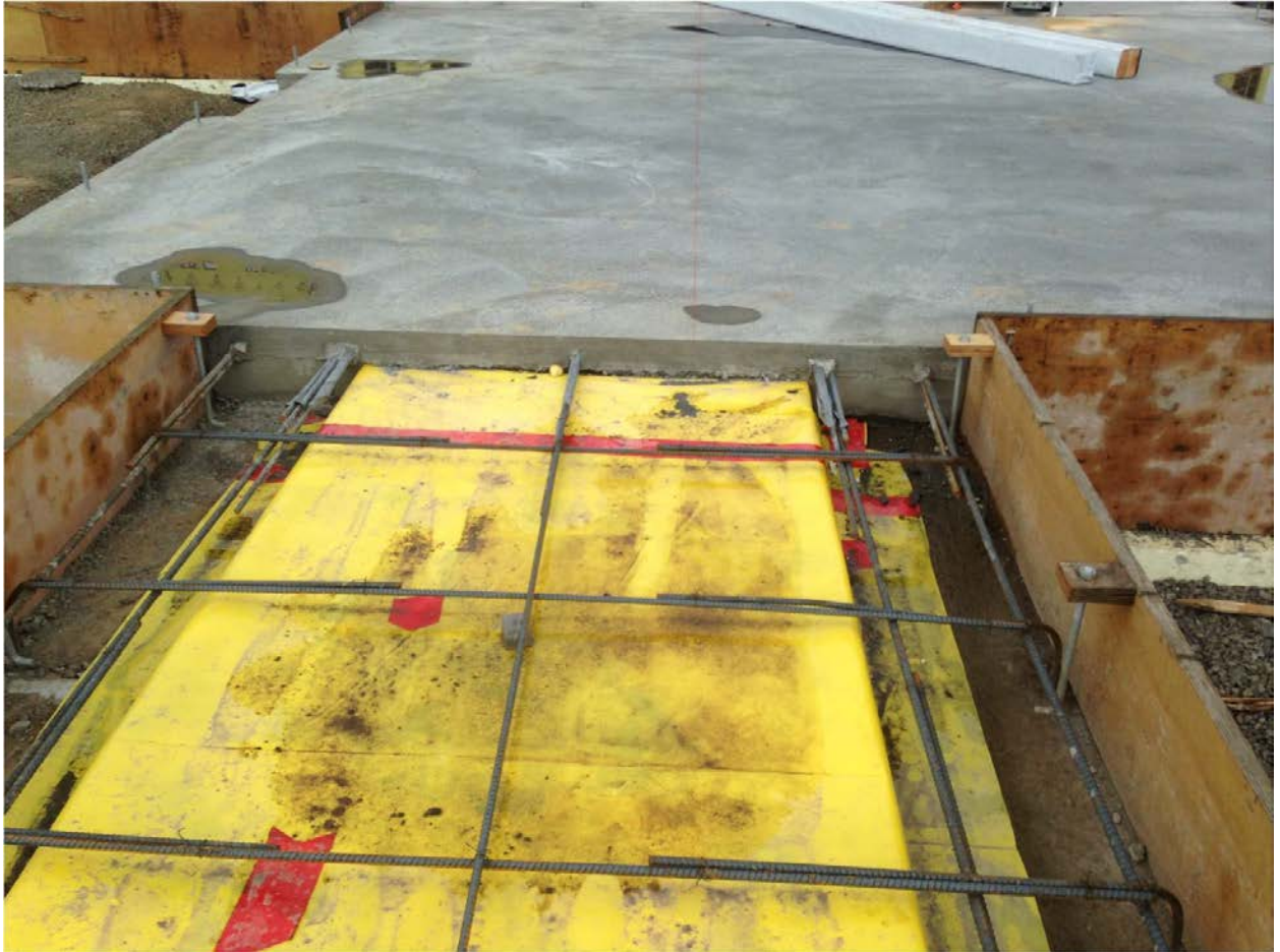
View of concrete slab and footings at the transition from Zone 1 (west wing) to Zone 2 (north wing).
