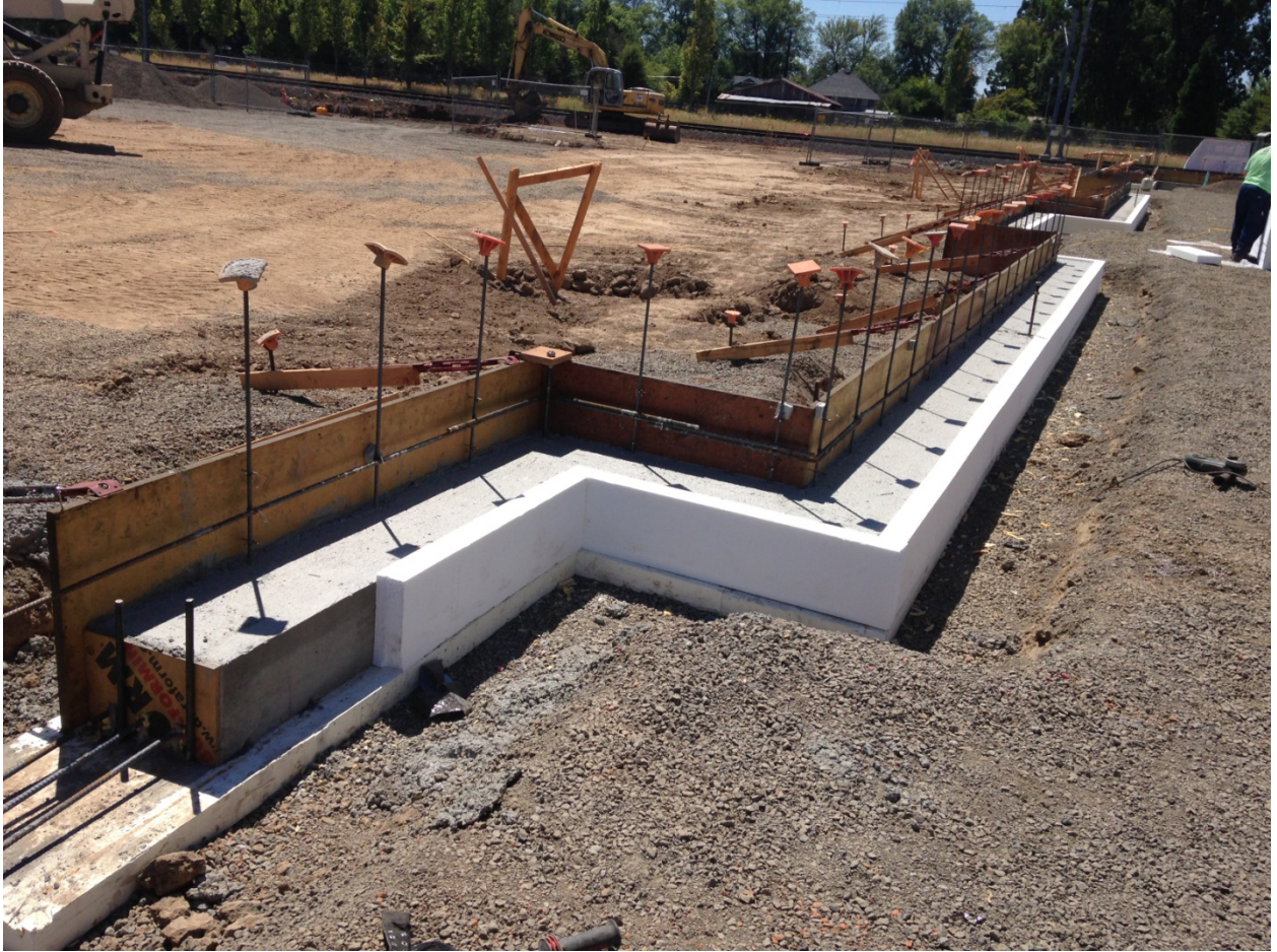
View of footing work in progress. Interior formwork has been stripped and foam is placed on the interior face of the footings.
