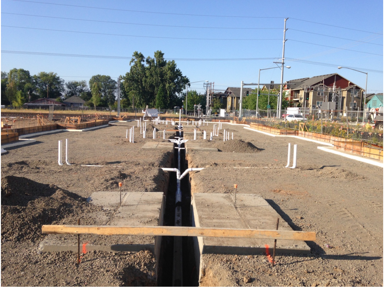
View of the Zone 1 (west wing) slab prep. The “deadman” footings that anchor hold downs for the seismic restraint system are visible in the foreground. The underground work for the plumbing system is also visible.
